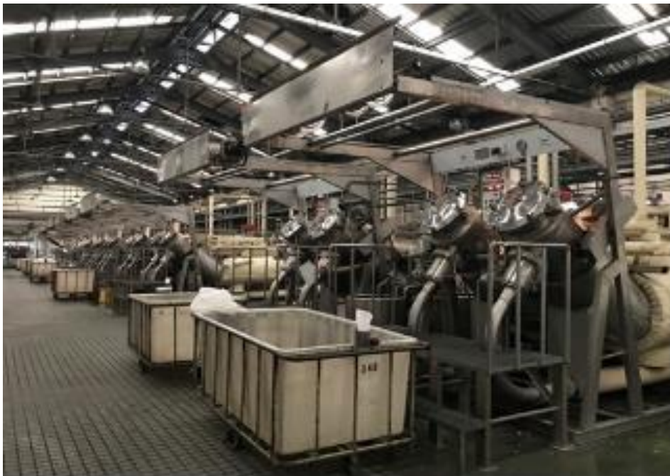
Figure 37 Textile Production Site at Viet Nam. No shopfloor data, low efficiency, lack of digital management and low productivity before digital transformation
