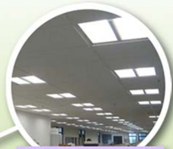
照明裝置 Lighting installation
