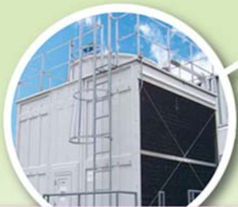
空調裝置 Air-conditioning installation
